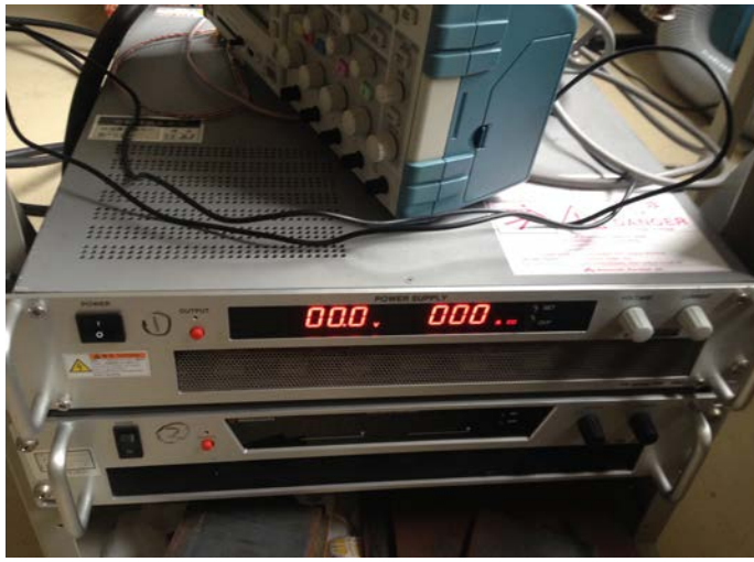
Fig. 37 DC current power supply.
